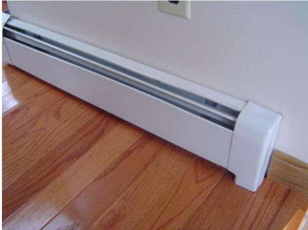
Electric Baseboard Wired
