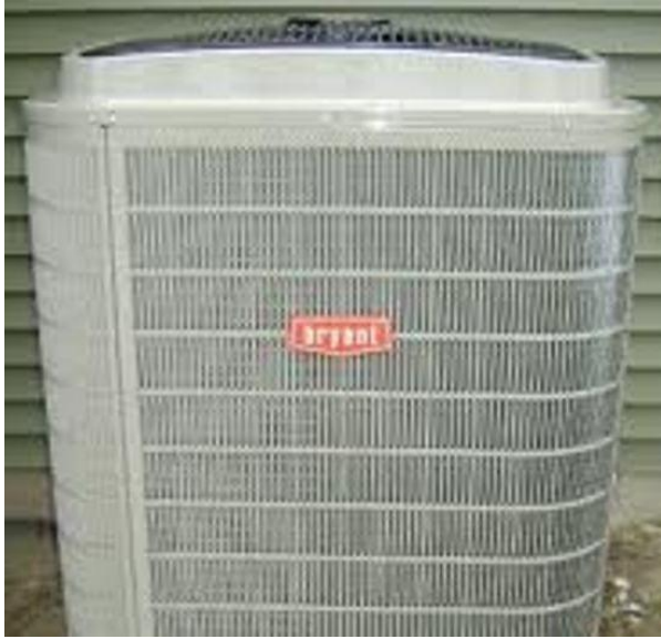
Condensing Unit (Heat Pump)
